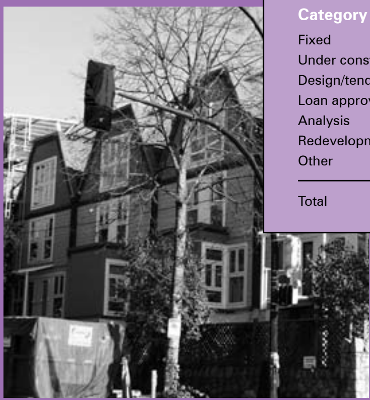
David Wetherow in Vancouver is one of six housing co-ops in the construction phase of building envelope repairs.
